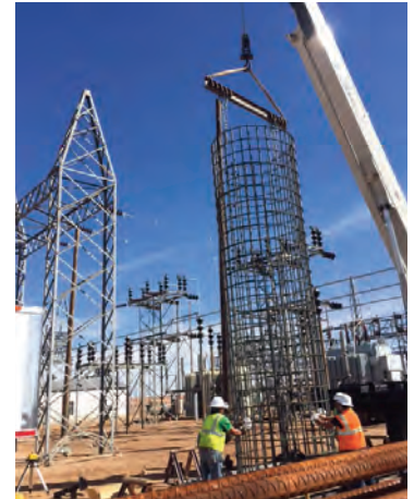
Crews construct a foundation on the China Draw-Wood Draw project south of Carlsbad.
