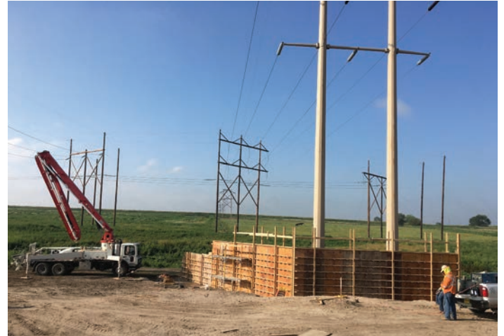
Crews work on building a retaining wall in preparation for upgrades being made at Deaf Smith Substation in Hereford, Texas.
