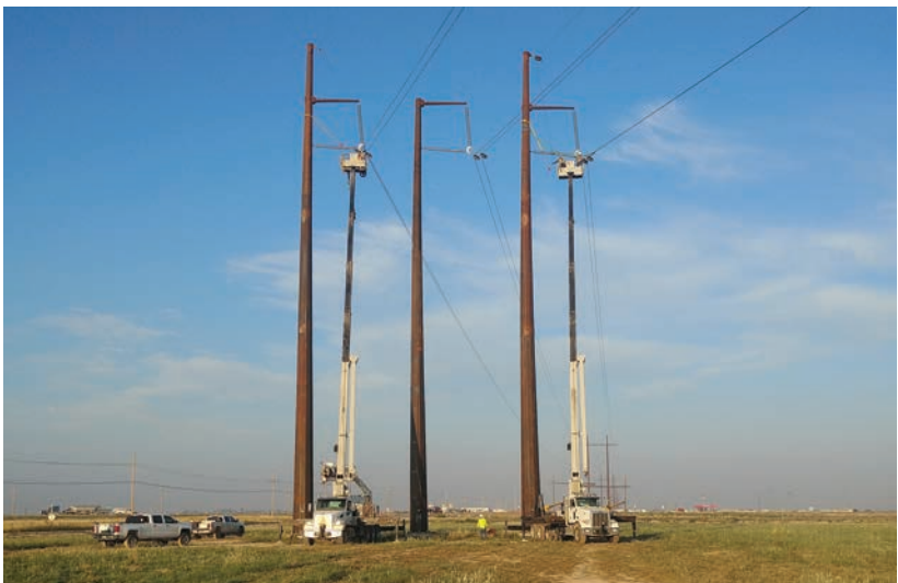
Construction is in full swing on the Hobbs-China Draw 345-kV transmission line. Crews work on clipping conductor on the line.
