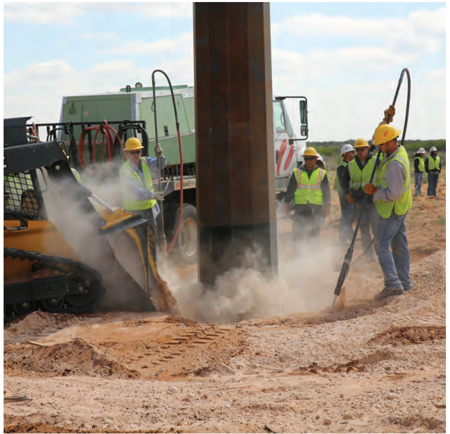
Crews tamp down a structure after setting it on the Potash Junction-Roadrunner line.
