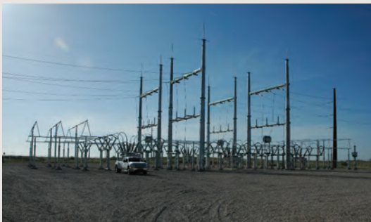
Quahada substation was energized in July 2015.
